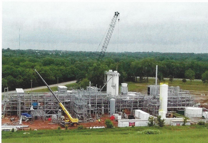
The ENVIA Energy GTL plant in Oklahoma City is progressing on schedule. (Source: Velocys)
