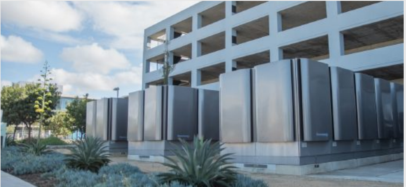
Copyright Bloom Energy, fuel cell system installed at a customer's corporate office, image used with permission
