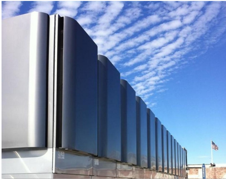
Adobe’s 400-kW fuel cell installation at its San Francisco office
