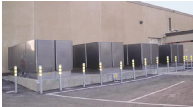
Cox’s 400 kW Bloom Energy installation in Oakland, California
