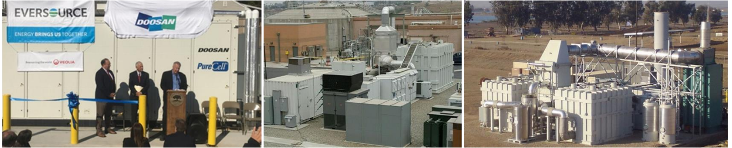
Figure 2. Doosan Fuel Cell America fuel cell at Naugatuck WWTP in Connecticut (L). FuelCell Energy fuel cell at Riverside WWTP in California (C). FuelCell Energy fuel cell at Tulare WWTP in California (R)
