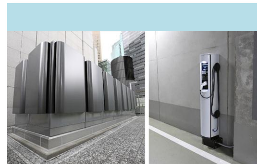
Tokyo Shiodome - Bloom Energy Server (left) supplies power to both the facility and the building's EV charging stations (right)
