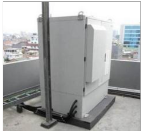
Ballard fuel cell system installed on rooftop
