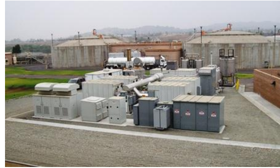
Fuel cell system located at an unspecified wastewater treatment plant.
