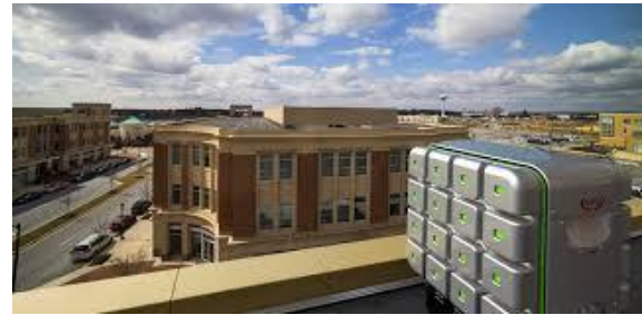
Redox Power Systems fuel cell sited on a roof.
