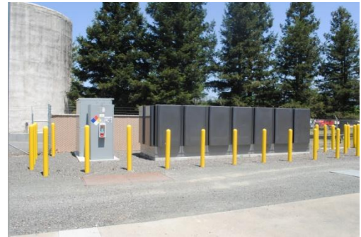
Bloom Energy installation at Sutter Home Winery.
