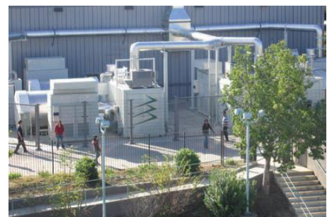
The California State University, Northridge subtropical rainforest (top image) uses wastewater from the fuel cell (bottom image) for irrigation
