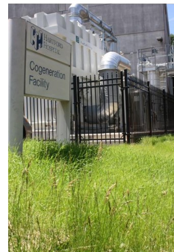
1.4 MW fuel cell power plant at Hartford Hospital in Connecticut
