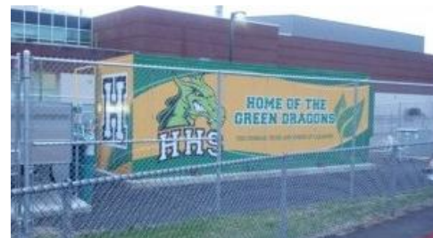
Hamden High School's fuel cell system (Hamden, Connecticut)
