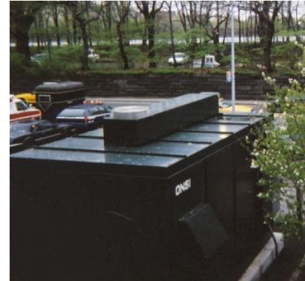
Fuel cell at Central Park Police Station in New York City.
