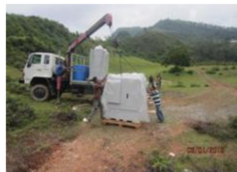
Ballard ElectraGen™-ME systems provide backup power for a telecom network in East Timor.
