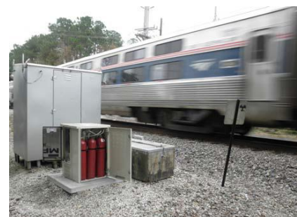
ReliOn E-200 fuel cells at a Florida railroad crossing.
