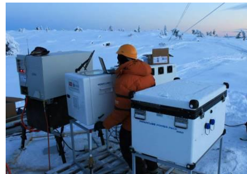
Acumentrics fuel cell at wind farm in Finland.
